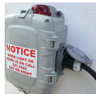
Generator Cord Connected
